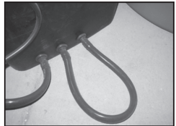
Unused outlets connected with tubing
